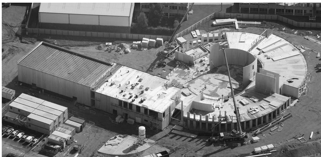
Slika 9. Izgradnja srednje škole u Noriču UK Figure 9. Construction of High School in Norwich, UK
